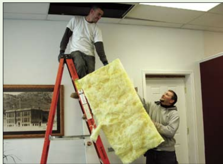
Photo by Emily Hanson Robert Lawrence handing insulation up to Jerry Degasperis at Inland Professional Title, LLC. Lawrence and Degasperis both work at Lawrence Construction Service which, on Monday, Dec. 15, was doing some interior renovations at Inland Professional Title, LLC. Lawrence said they were replacing an exterior door and insulating the building.
